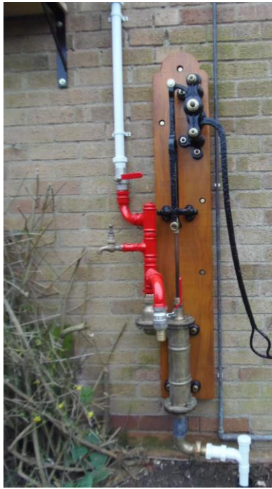
Pump & Header Tank
